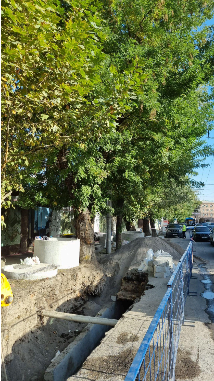
Figure 2: Evidence of Undermining Structural undermining of Tree #3.
